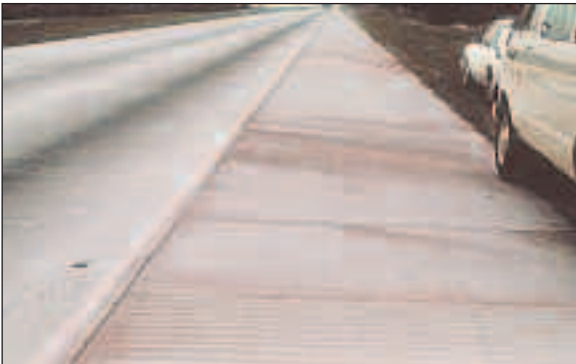
Figure 131: Distress Type CRCP 14 Water Bleeding and Pumping
