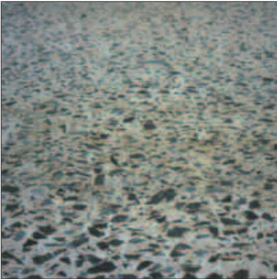
Figure 103: Distress Type CRCP 5 Polished Aggregate
