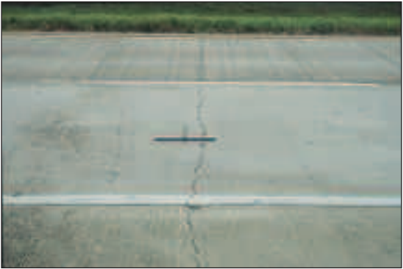
Figure 99: Distress Type CRCP 3 Moderate Severity Transverse Cracking
