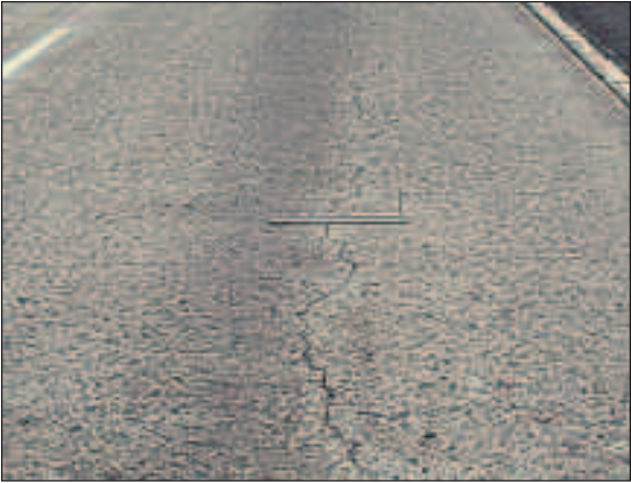
Figure 94: Distress Type CRCP 2 Low Severity Longitudinal Cracking
