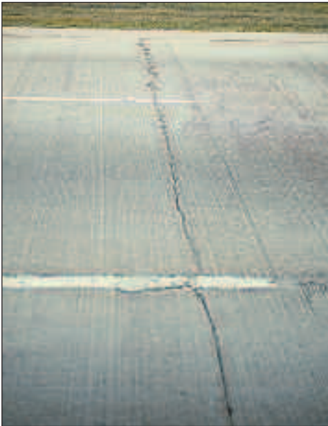
Figure 112: Distress Type CRCP 8 – Moderate Severity Transverse Construction Joint Deterioration
