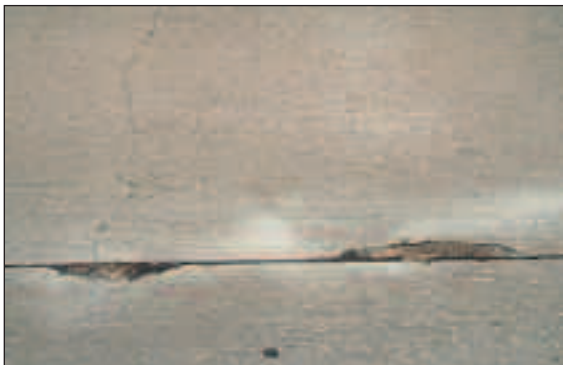
Figure 130: Distress Type CRCP 13 - Close-up View Moderate Severity Spalling of Longitudinal Joints
