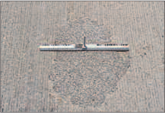
Figure 119: Distress Type CRCP 11 Small, Low Severity Asphalt Concrete Patch
