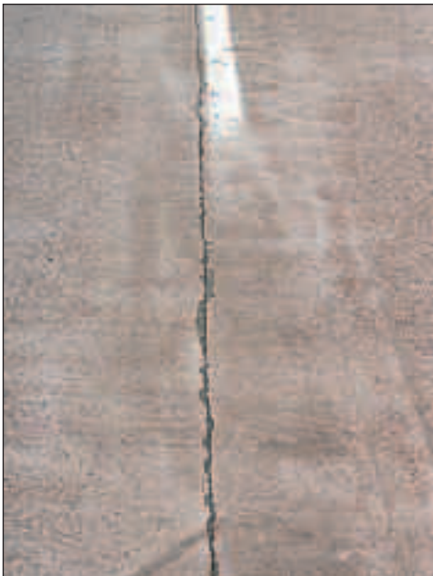
Figure 129: Distress Type CRCP 13 Low Severity Spalling of Longitudinal Joints
