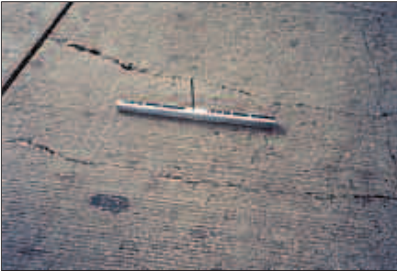
Figure 124: Distress Type CRCP 12 Low Severity Punchouts
