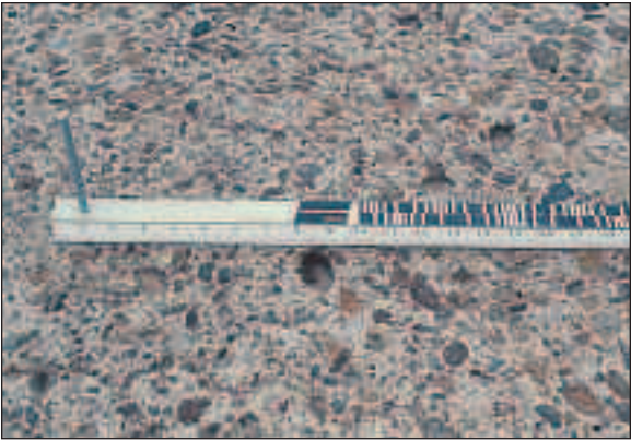
Figure 105: Distress Type CRCP 6 - Popouts
