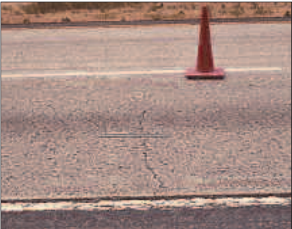
Figure 98: Distress Type CRCP 3 Low Severity Transverse Cracking
