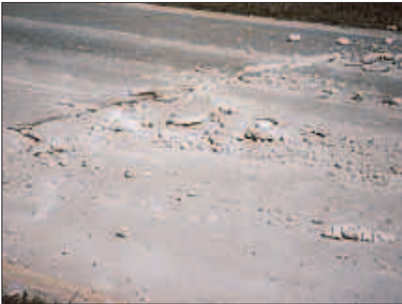
Figure 107: Distress Type CRCP 7 – A Blowup
