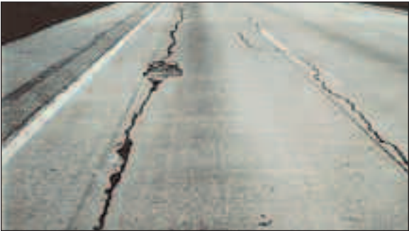
Figure 95: Distress Type CRCP 2 High Severity Longitudinal Cracking
