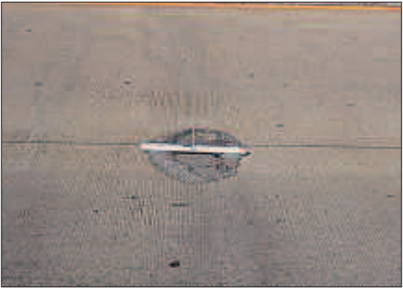
Figure 121: Distress Type CRCP 11 Moderate Severity Asphalt Concrete Patch
