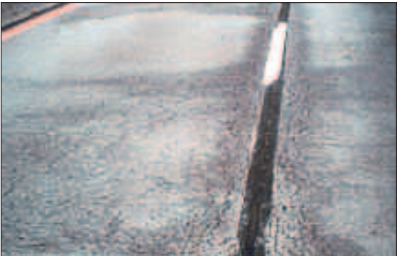
Figure 92: Distress Type CRCP 1 High Severity “D” Cracking at Longitudinal Joint
