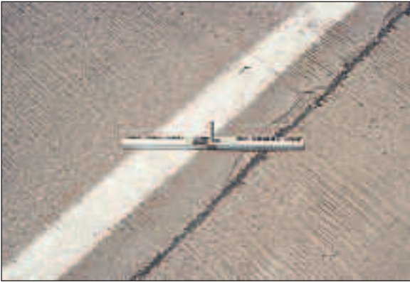
Figure 128: Distress Type CRCP 13 - Close-up View Low Severity Spalling of Longitudinal Joints
