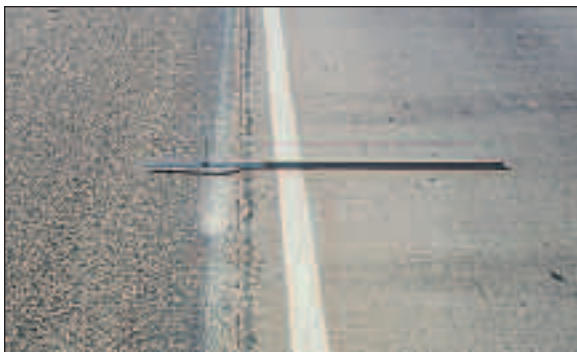
Figure 115: Distress Type CRCP 9 Lane-to-Shoulder Dropoff
