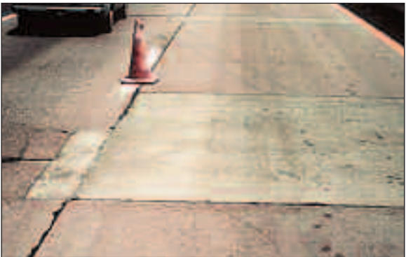
Figure 122: Distress Type CRCP 11 Low Severity Portland Cement Concrete Patch
