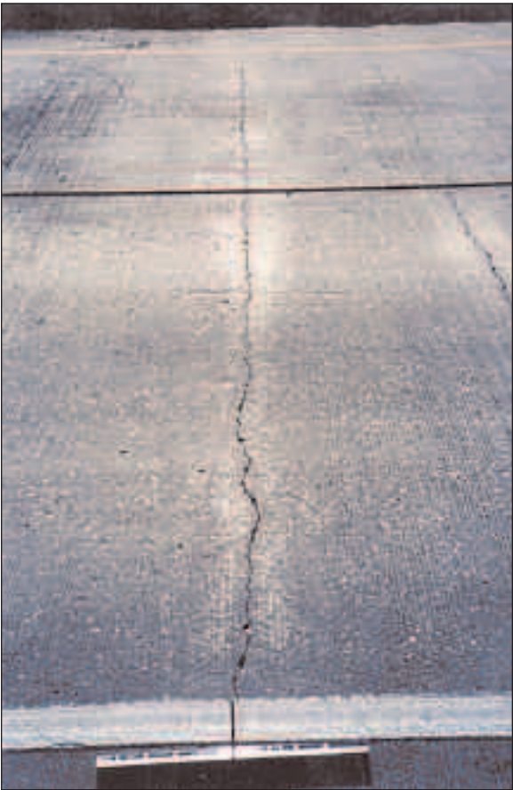
Figure 113: Distress Type CRCP 8 – Low Severity Transverse Construction Joint Deterioration
