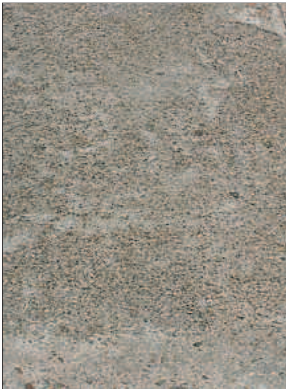
Figure 102: Distress Type CRCP 4b - Scaling
