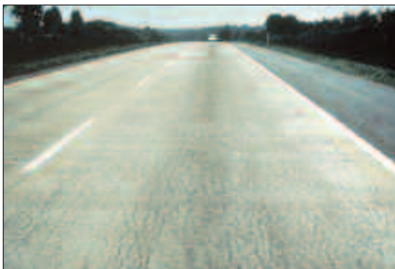
Figure 101: Distress Type CRCP 4a Map Cracking Attributable to Alkali-Silica Reactivity
