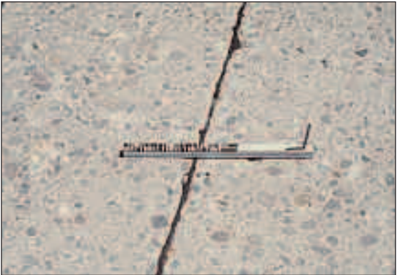
Figure 62: Distress Type JCP 5 Moderate Severity Joint Seal Damage
