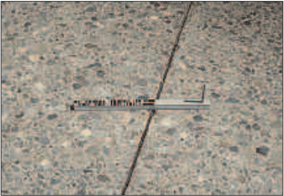
Figure 61: Distress Type JCP 5 Low Severity Joint Seal Damage
