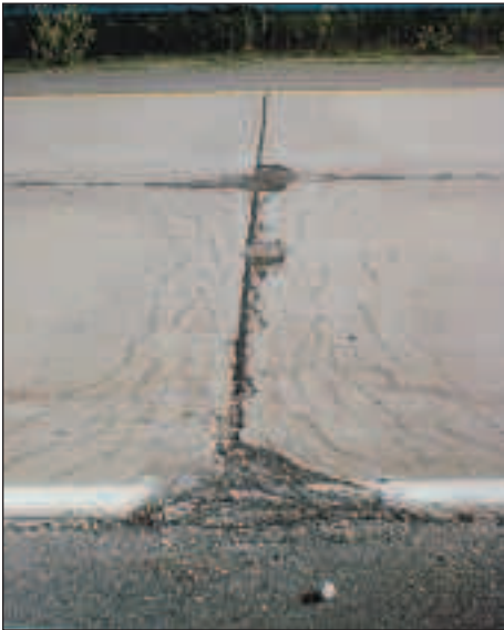
Figure 53: Distress Type JCP 2 High Severity “D” Cracking with Loose and Missing Material
