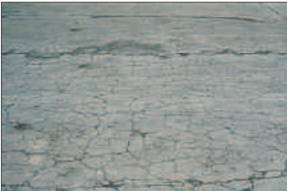
Figure 69: Distress Type JCP 8a – Map Cracking
