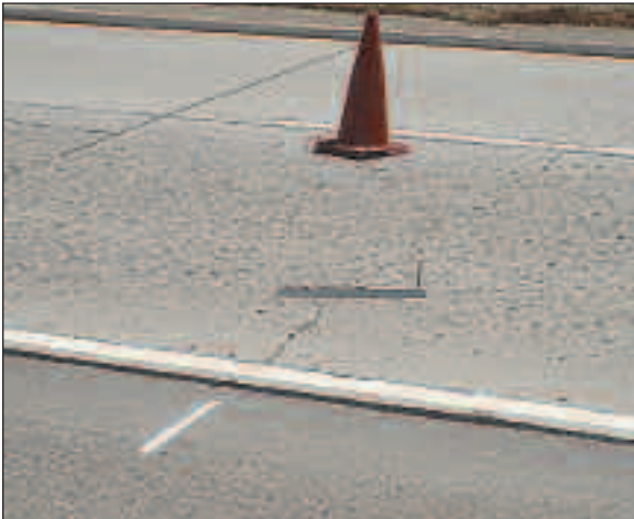
Figure 59: Distress Type JCP 4 Moderate Severity Transverse Cracking
