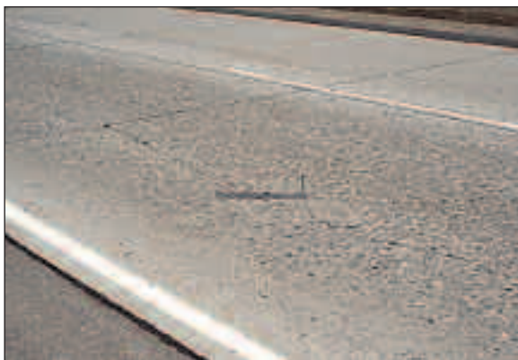
Figure 56: Distress Type JCP 3 Moderate Severity Longitudinal Cracking
