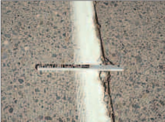
Figure 64: Distress Type JCP 6 Low Severity of Longitudinal Joint
