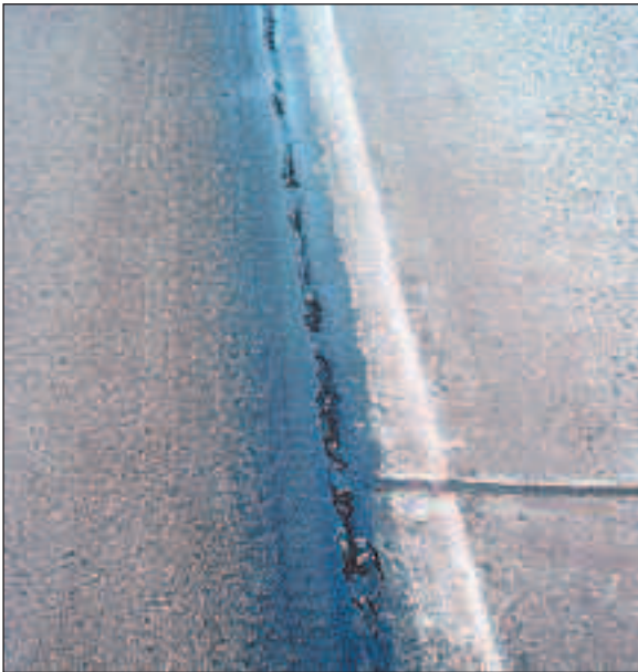
Figure 82: Distress Type JCP 14 Poorly Sealed Lane-To-Lane Separation
