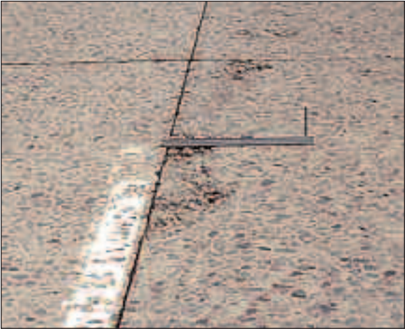
Figure 65: Distress Type JCP 6 High Severity Spalling of Longitudinal Joint
