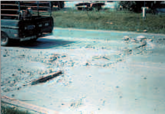
Figure 76: Distress Type JCP 11 – A Blowup
