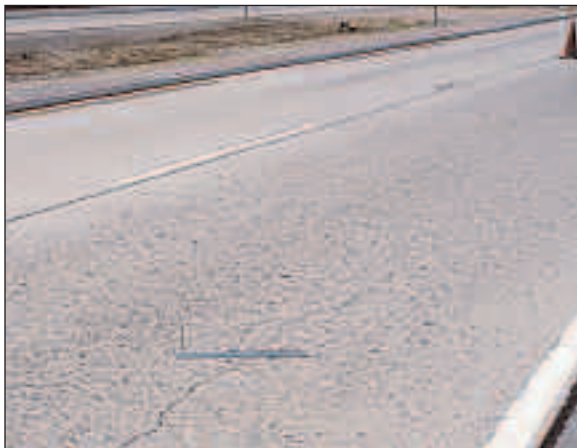
Figure 55: Distress Type JCP 3 Low Severity Longitudinal Cracking
