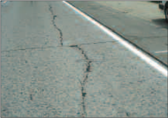
Figure 57: Distress Type JCP 3 High Severity Longitudinal Cracking
