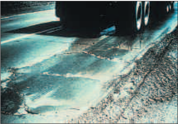
Figure 89: Distress Type JCP 16 Water Bleeding and Pumping
