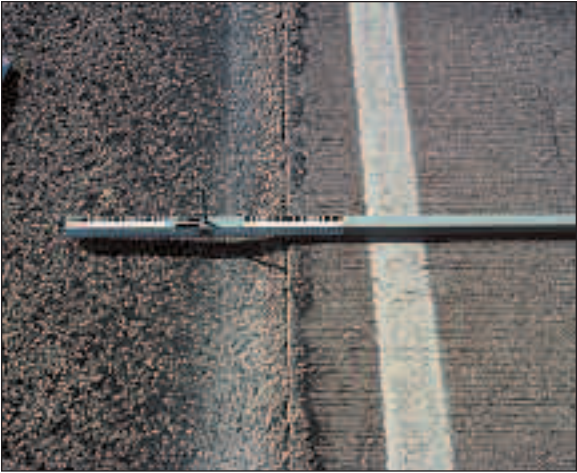
Figure 80: Distress Type JCP 13 Lane-To-Shoulder Dropoff
