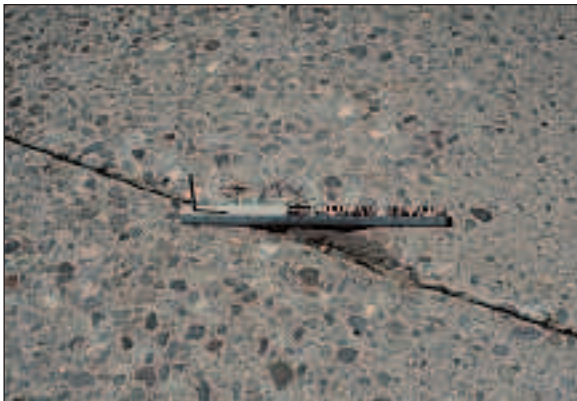
Figure 68: Distress Type JCP 7 Moderate Severity Spalling of Transverse Joint Close-up View
