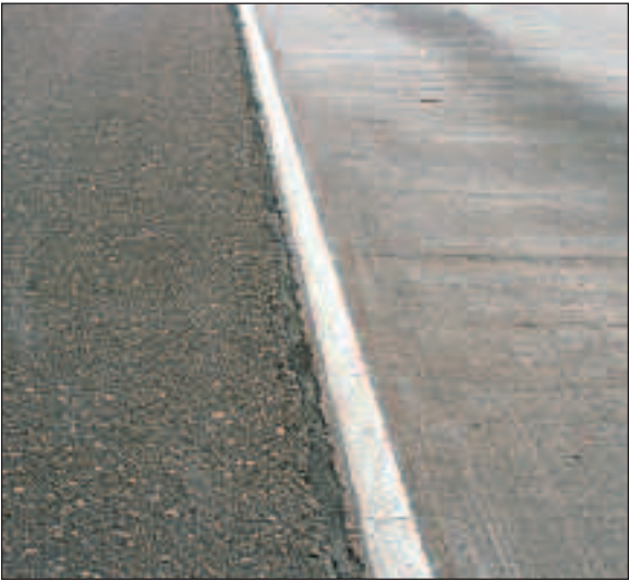
Figure 83: Distress Type JCP 14 Well Sealed Lane-To-Lane Separation
