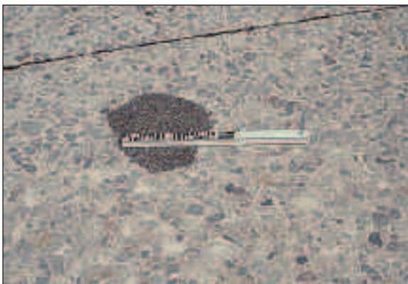
Figure 85: Distress Type JCP 15 Small, Low Severity Asphalt Concrete Patch
