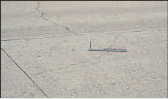
Figure 49: Distress Type JCP 1 Low Severity Corner Break
