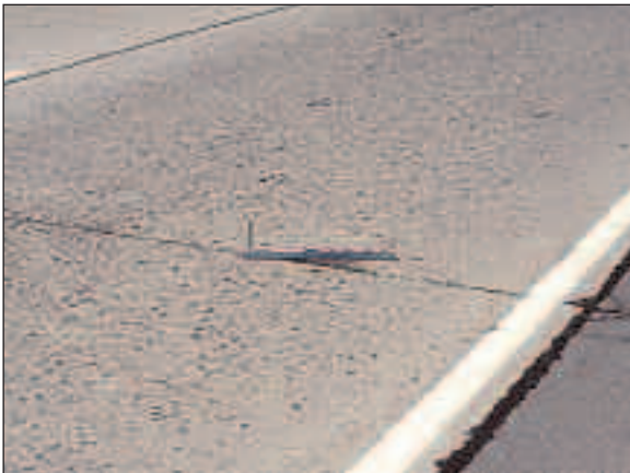
Figure 67: Distress Type JCP 7 Moderate Severity Spalling of Transverse Joint Far View
