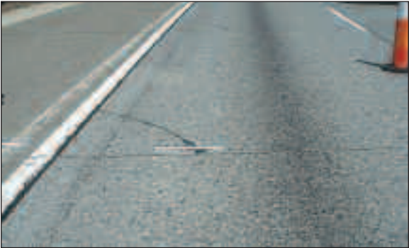
Figure 50: Distress Type JCP 1 Moderate Severity Corner Break
