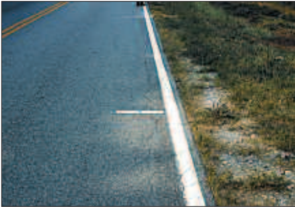
Figure 12: Distress Type ACP 3 Low Severity Edge Cracking
