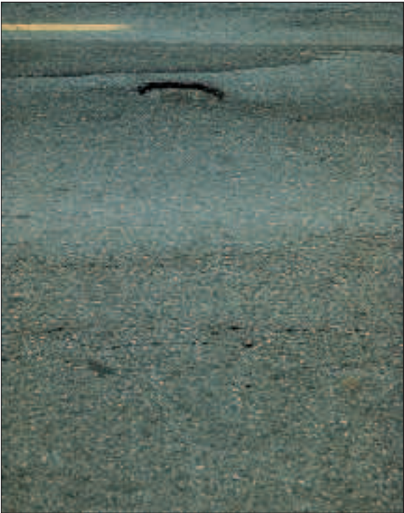
Figure 28: Distress Type ACP 8 Moderate Severity Pothole
