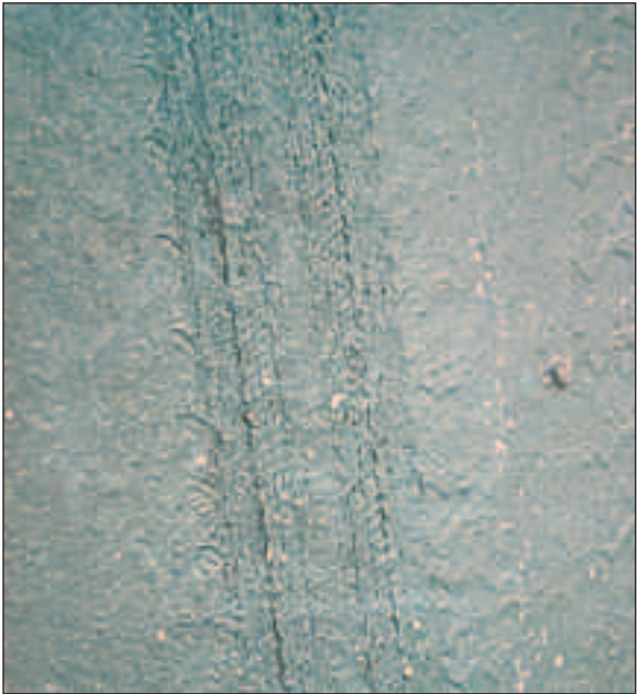
Figure 38: Distress Type ACP 11 High Severity - Aggregate Obscured
