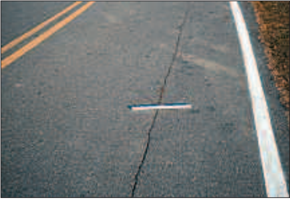
Figure 14: Distress Type ACP 4a Moderate Severity Longitudinal Cracking in the Wheel Path
