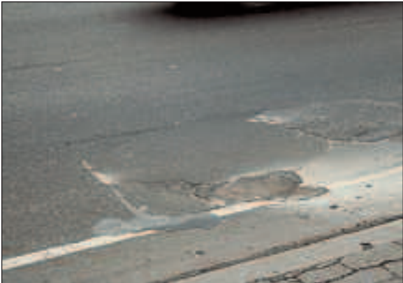
Figure 25: Distress Type ACP 7 High Severity Patch
