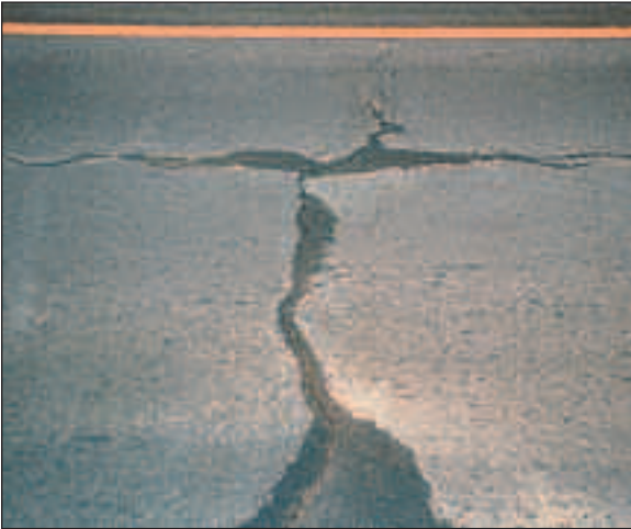
Figure 45: Distress Type ACP 15 Water Bleeding and Pumping
