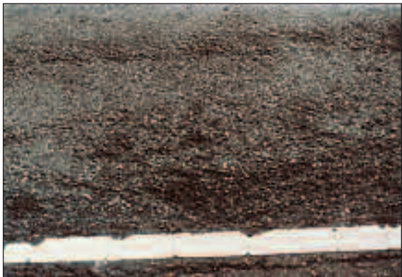
Figure 41: Distress Type ACP 13 – Moderate Severity Loss of Fine and Some Coarse Aggregate
