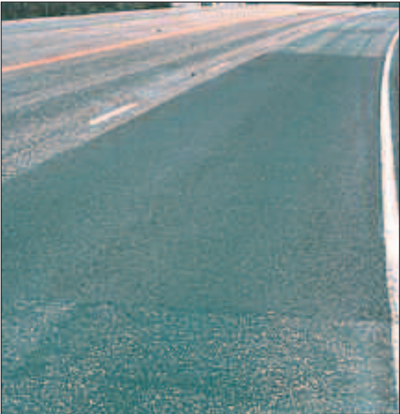
Figure 23: Distress Type ACP 7 Low Severity Patch
