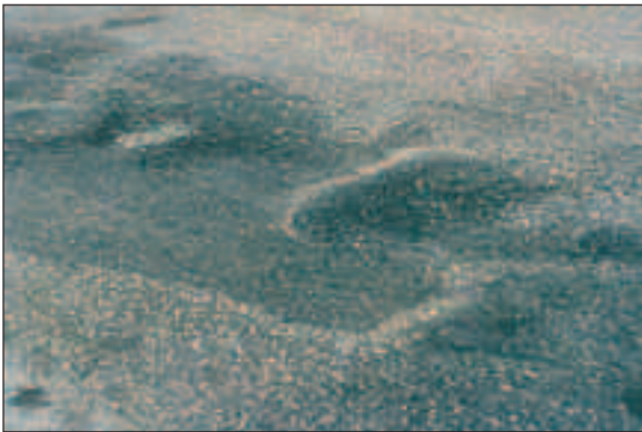
Figure 35: Distress Type ACP 10 Shoving in Pavement Surface
