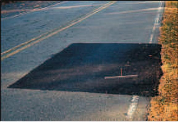
Figure 24: Distress Type ACP 7 Moderate Severity Patch
