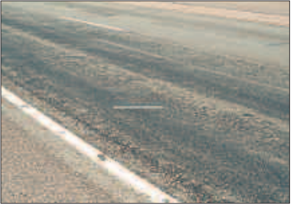
Figure 37: Distress Type ACP 11 Moderate Severity - Loss of Texture
