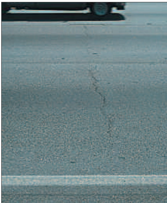
Figure 19: Distress Type ACP 6 Low Severity Transverse Cracking
