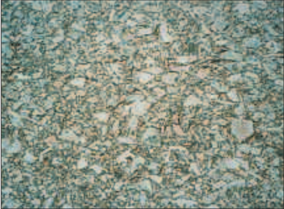
Figure 39: Distress Type ACP 12 - Polished Aggregate
