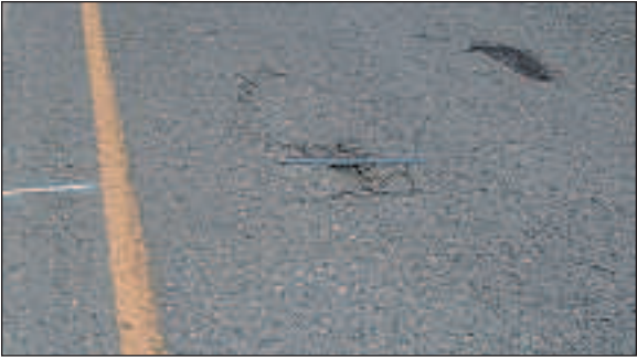
Figure 27: Distress Type ACP 8 Low Severity Pothole
