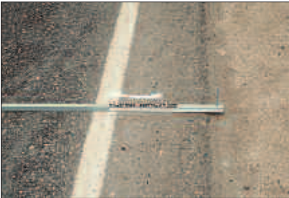
Figure 44: Distress Type ACP 14 Lane-to-Shoulder Dropoff
