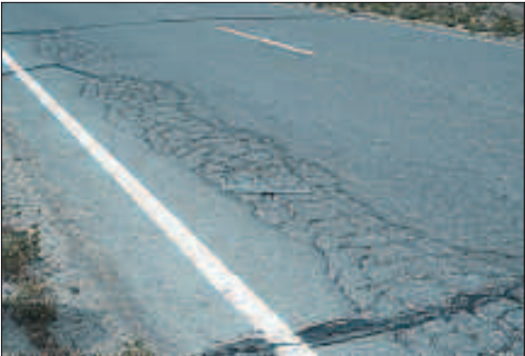
Figure 7: Distress Type ACP 1 High Severity Fatigue Cracking with Spalled Interconnected Cracks
