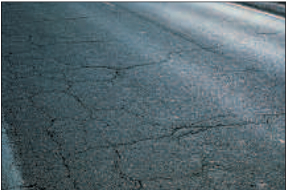
Figure 10: Distress Type ACP 2 High Severity Block Cracking
