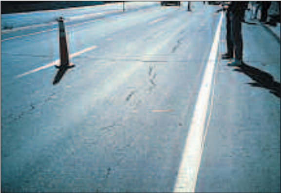
Figure 5: Distress Type ACP 1 - Low Severity Fatigue Cracking
