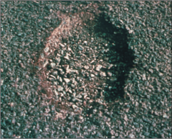
Figure 29: Distress Type ACP 8 Moderate Severity Pothole, Close-up View
