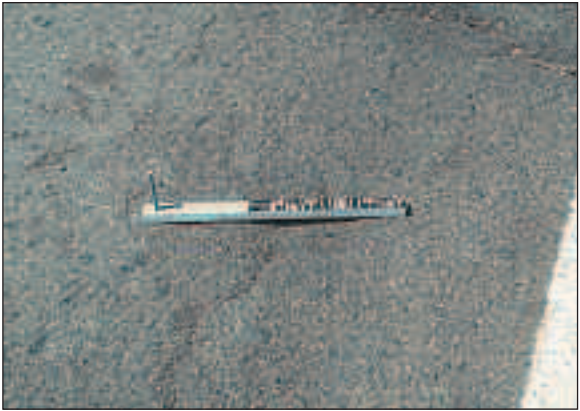
Figure 40: Distress Type ACP 13 Low Severity - Loss of Fine Aggregate
