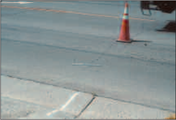
Figure 20: Distress Type ACP 6 Moderate Severity Transverse Cracking
