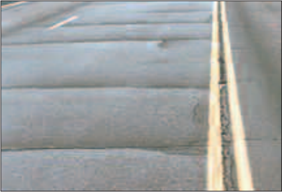
Figure 17: Distress Type ACP 5 High Severity Reflection Cracking at Joints
