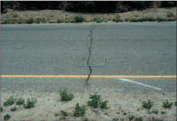
Figure 21: Distress Type ACP 6 High Severity Transverse Cracking
