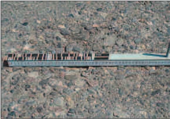
Figure 42: Distress Type ACP 13 Loss of Coarse Aggregate
