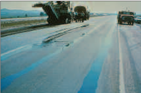
Figure 33: Distress Type ACP 9 Standing Water in Ruts
